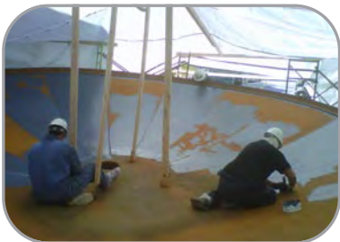
Mining project requiring metal resurfacing and rubber relining of 25' dia process tank.
